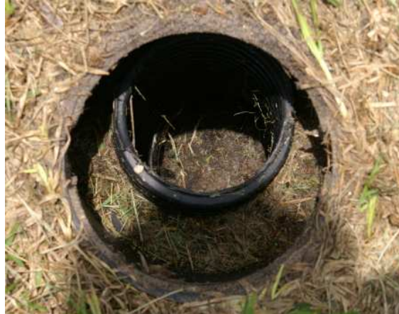
Sight tube at upper layer of ADS multi-pipe system.
