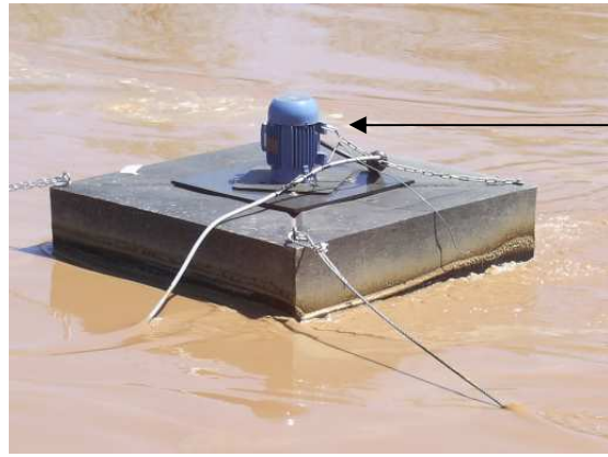
VBT™ on Float in Oxidation Ditch
