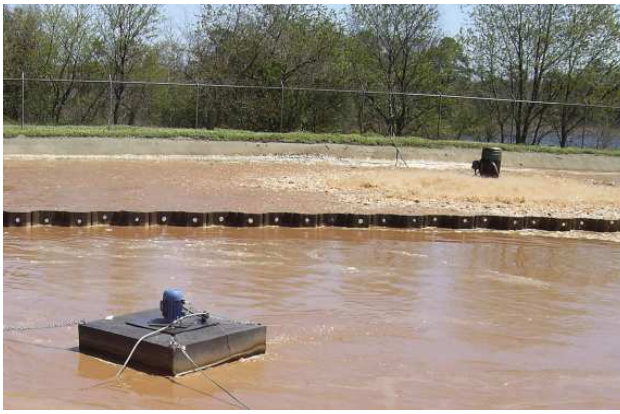
VBT™ and Surface Aerator in Oxidation ditch
